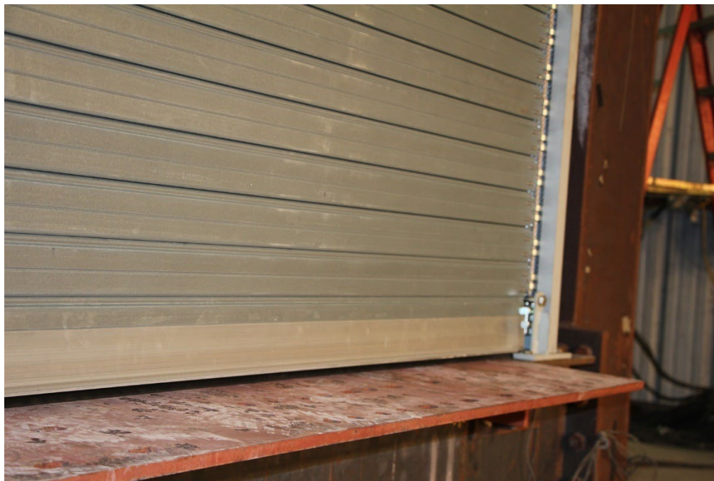
Figure 20. View of Curtain Sill – PL 2 Configuration
